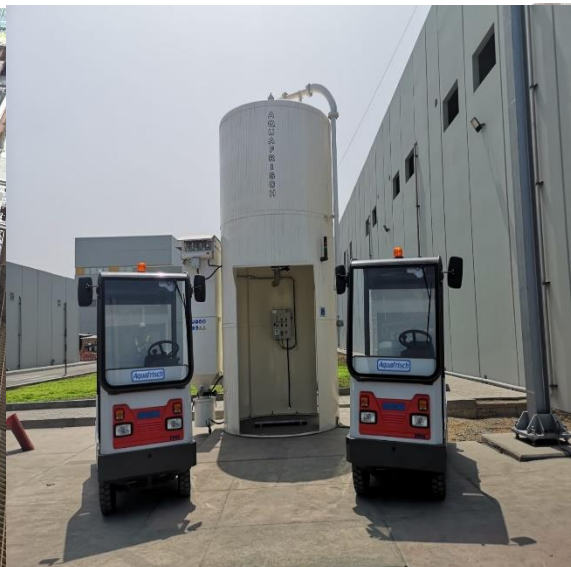
Mobil Sand Dispenser and Silo at Lima (Peru)
